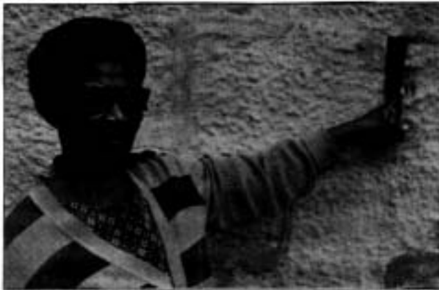
Mrs Luthuli of the Women's Group shows an unrepaired hole in a house in Lamontville.
